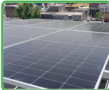
10 KW Plant, Anandham
