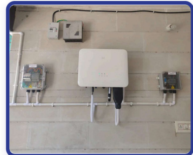
Inverter & Electrical Setup
