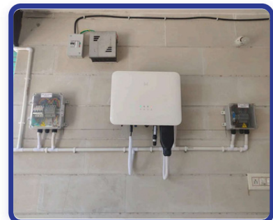
Inverter & Electrical Setup
