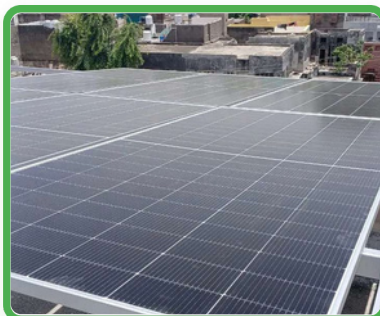
10 KW Plant, Anandham
